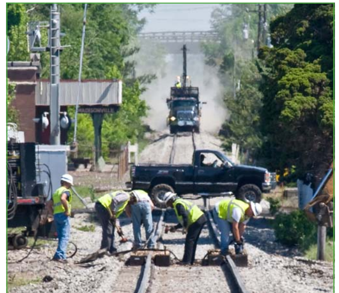
A CSX MOW crew works on repaving the crossing at West Broadway Street, Madisonville, Ky on Wednesday, May 5th, 2010 during the current right-of-way upgrades on the Henderson Subdivision. (Photo by Jim Pearson)
